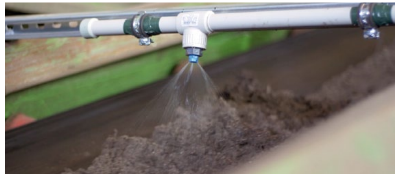
Spray nozzles above the conveyor belt wet the substrate
